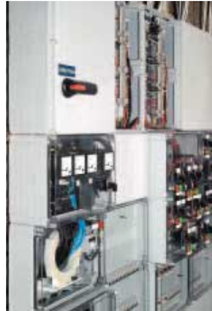
This Cubo P of a sewage treatment plant is a wide system of 33 enclosures.
