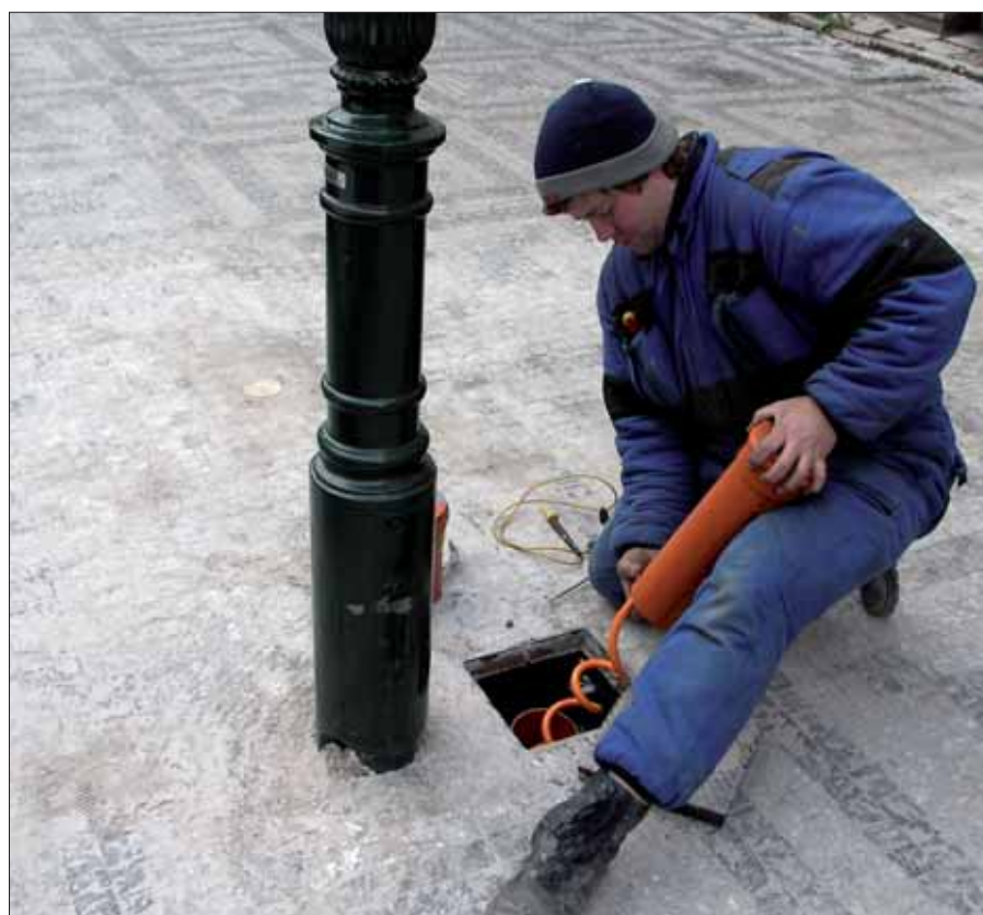
The application of UFK D125 as a connection point for electrical control of solenoid in a gas lamp pole.
